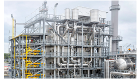
(c) Gas-fired boiler plant
